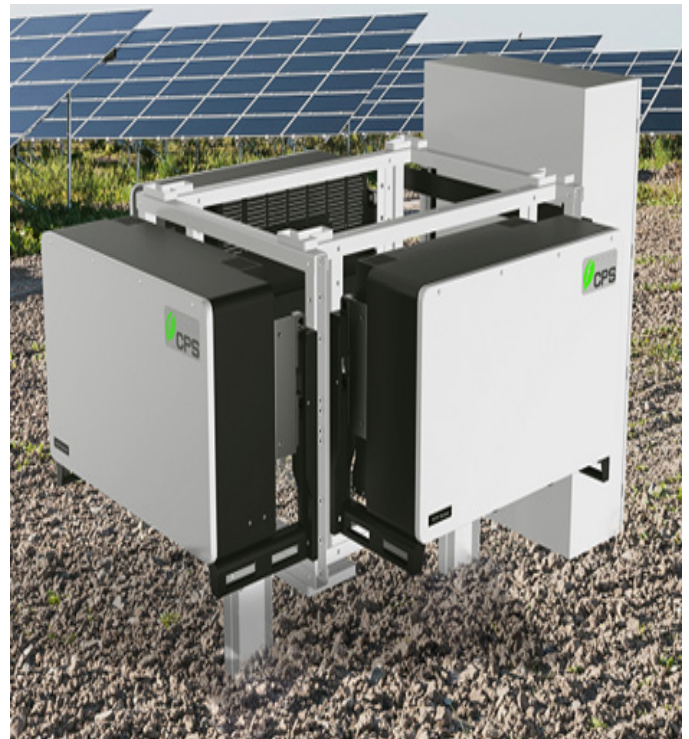
(3) CPS 250/275kW Inverters + (1) CPS 800V AC Combiner Installed with Cluster Mounting Bracket
