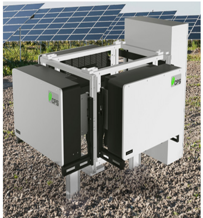
(3) CPS 250/275kW Inverters + (1) CPS 800V AC Combiner installed with Cluster Mounting Bracket
